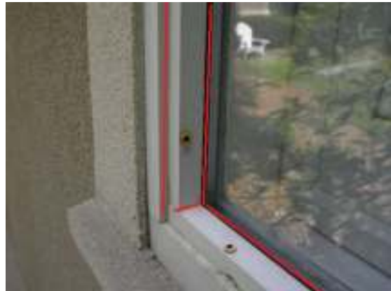
A This type of fixed glass window should be sealed (wet glazed)
