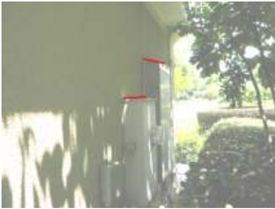
A. Insure all utility fixtures are sealed.
