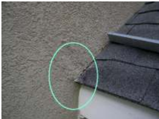
B. Missing kickout flashing detail.
