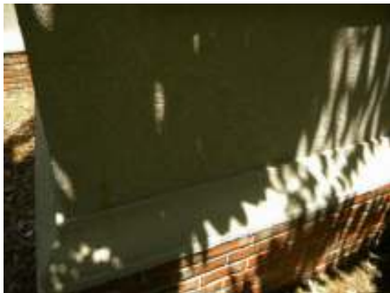
B. Random minor cracks in the stucco cap band
