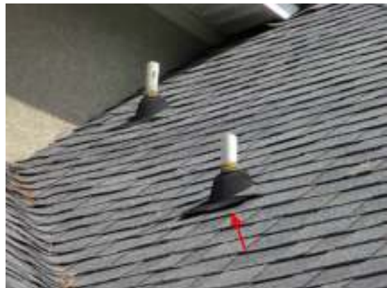
C. Vent boots here need fastened.
