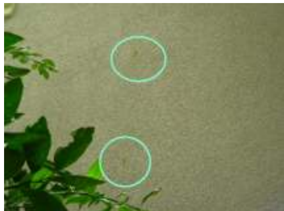
Misc. Some rust aggregate in stucco finish thru out the system.
