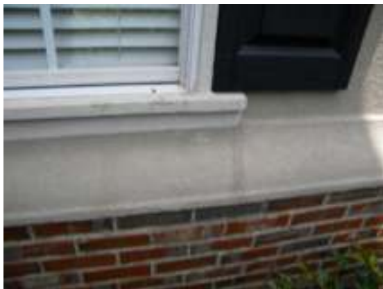
Minor band cracking at a few locations
